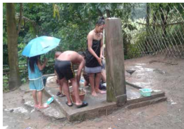
Figure 33 - Deep well with handpump in Samuoi District UN-Habitat, 2017
