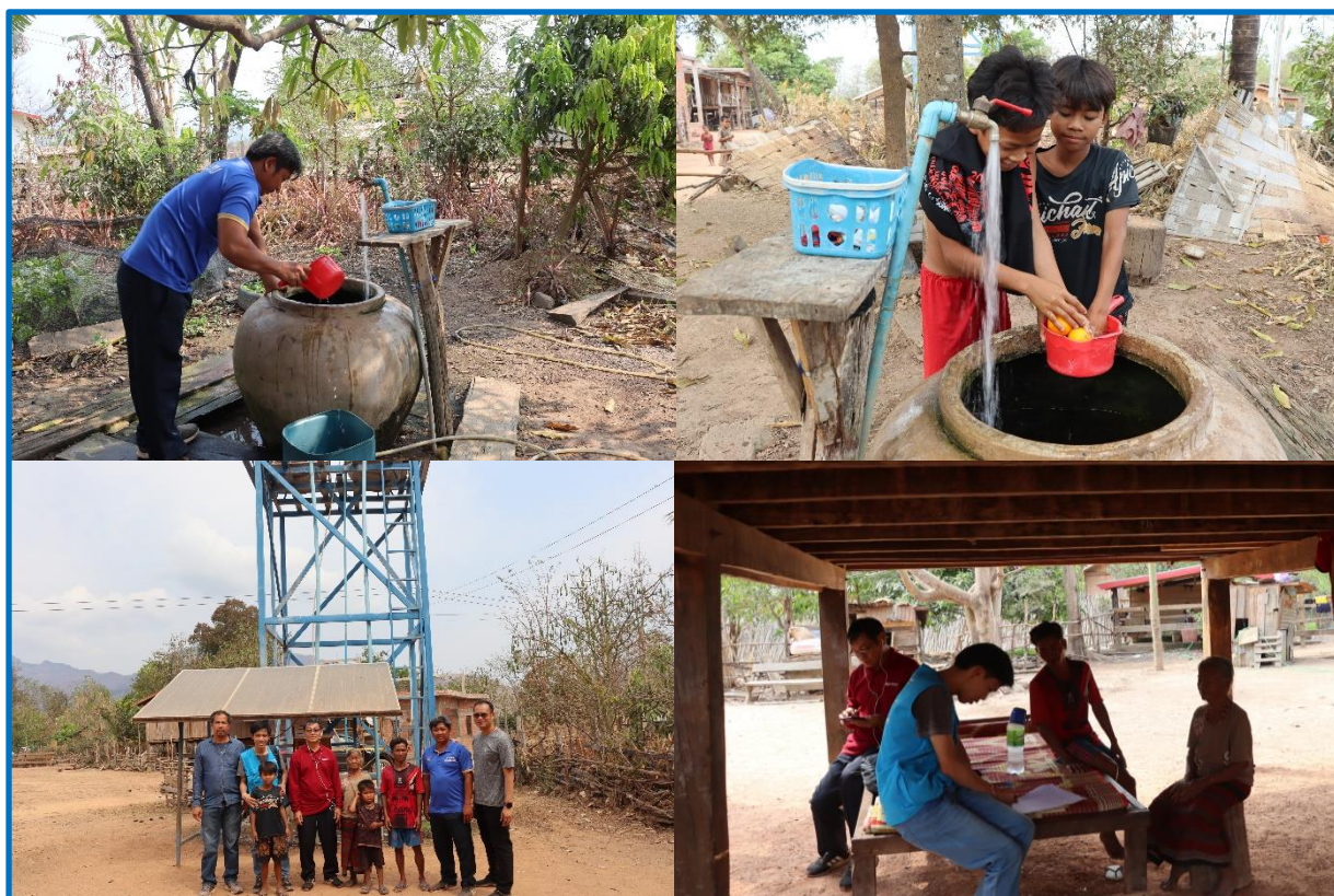
Figure 3: Operational Assessment - Borehole-Over-head tanks (with solar panel) water supply system in Sanyayon village, Ta-oy, Saravane Province
