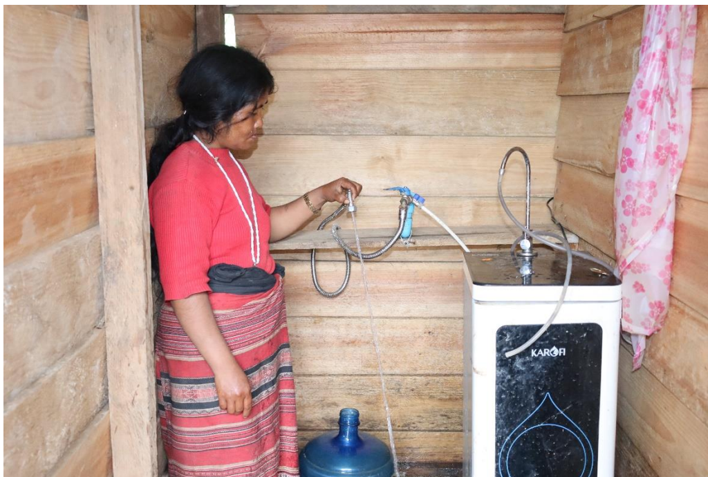
Figure 10: Operational Assessment – a newly built toilet with water connection to the toilet in Daksa Village, Dakcheung district, Sekong province.
