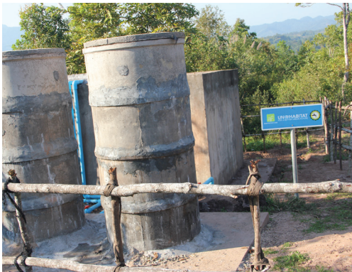
Water tank with slow sand filter system, Tangko village, Samuoi District, Saravane Province, 2020. (Photo by UN-Habitat / Juan A. Torres)
